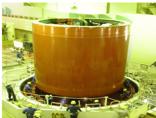
Photograph: Rotor of 400 MW, 330-390 min-1, 700 tons, 6000 mm, asynchronous generator-motor
