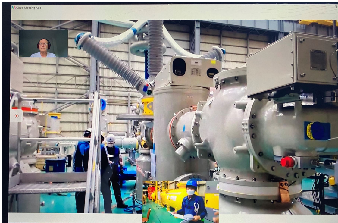
Figure 3 - Ongoing routine tests on manufacturer side of HV switchgear. Camera view from tester's hard hat.
